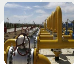
City Gas Distribution
